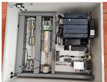
Fire Station Alerting control box after installation.
