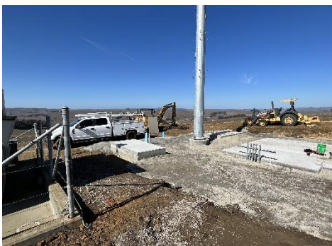
Monopole base at Tomales site.
